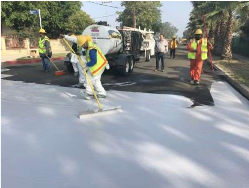
Figure 36. Lighter pavement surfaces like this one do not retain as much heat as conventional pavement treatments.
