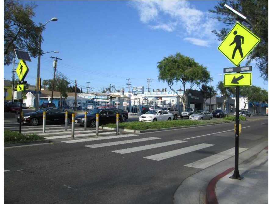
Figure 37. Rectangular Rapid Flashing Beacons (RRFBs) are an option for upgrading unsignalized pedestrian crossings.
