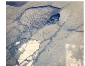
Poor pavement quality in a bicycle lane
