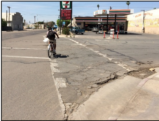
Figure 6-8: Poorly maintained roadway infrastructure along Fifth Street
