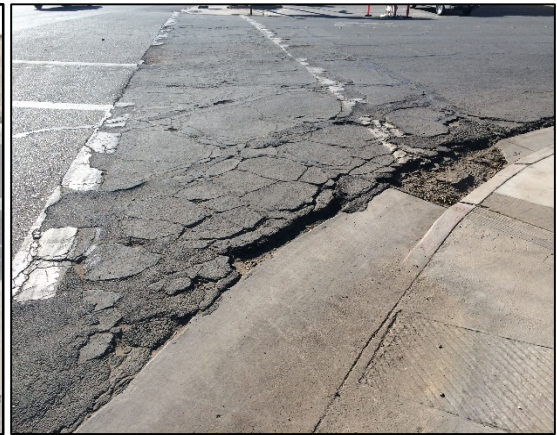
Figure 4-7: Poor crosswalk condition around Holt Park
