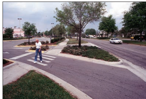
Right turn only driveway with a splitter island simplifies turning movements and facilitates pedestrian crossing.
