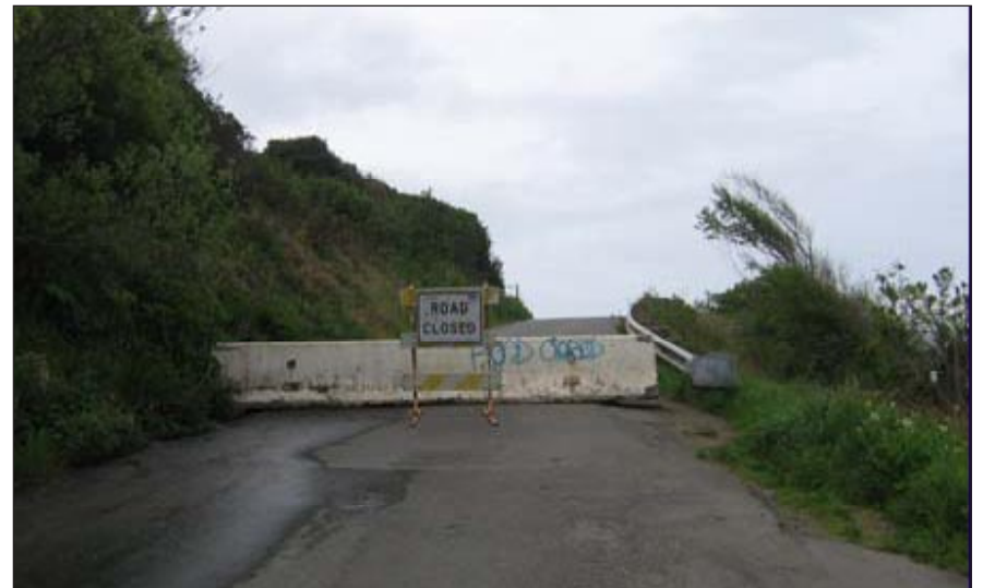
Road closure after 2006 winter storm
