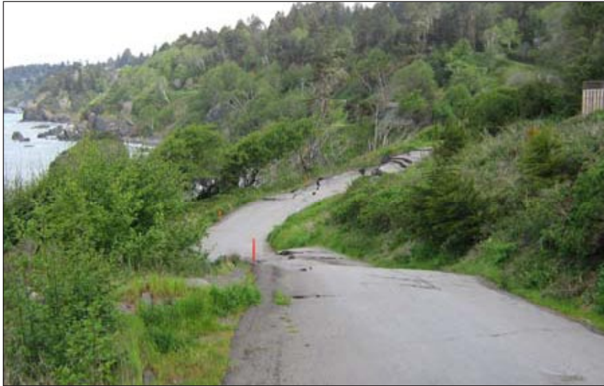
330 feet of impassible road
