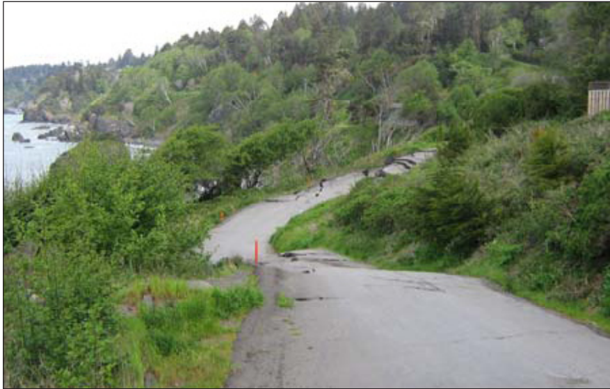
330 feet of impassible road
