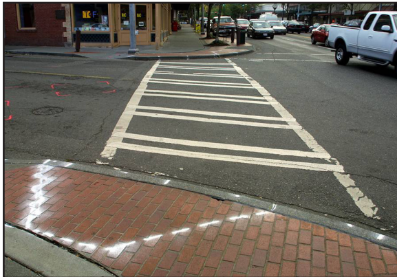
ADA requirements were often originally met in haste without proper alignment of paths. Many municipalities are now correcting these placements.
