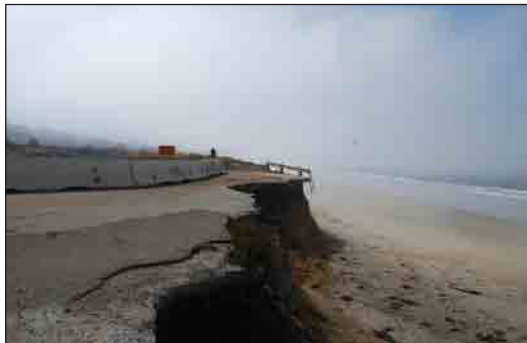
Erosion destroyed old roadways through El Granada and continues to move toward Highway 1.
