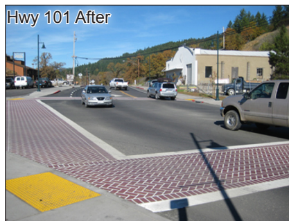
High contrast pavement treatment to highlight the pedestrian crossing area is added to an intersection on Highway 101.
