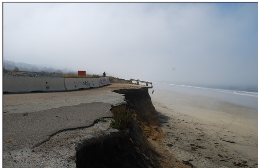
Erosion destroyed old roadways through El Granada and continues to move toward Highway 1.
