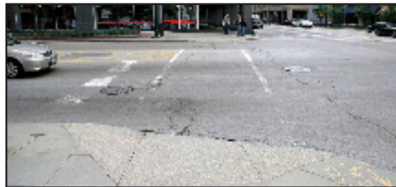
Crossing enhancements (especially stripes) should be maintained to draw motorist attention to pedestrian zones. Crossings that are not maintained lead to less certain (and less visible) pedestrian paths.
