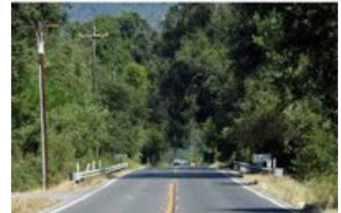
Hwy 162 bridge crossing Mill Creek has narrow shoulders.
