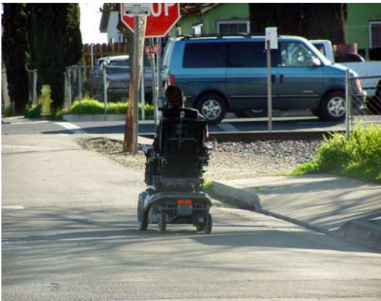
Curb ramps should be designed so that people with mobility and vision limitations can use the sidewalk system.
