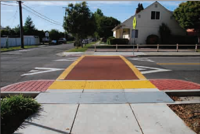
View of the crosswalk from a pedestrian perspective. Note that the curb extensions were constructed separated from the existing curb to preserve existing drainage.
