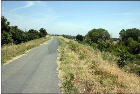
The recreational trail on this levee in Marysville has few connections with downtown or other destinations.
