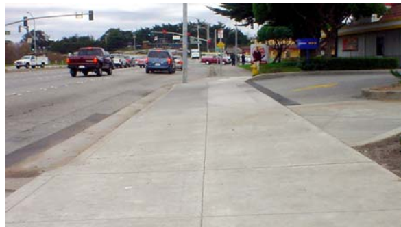
New driveway with no flat area.
