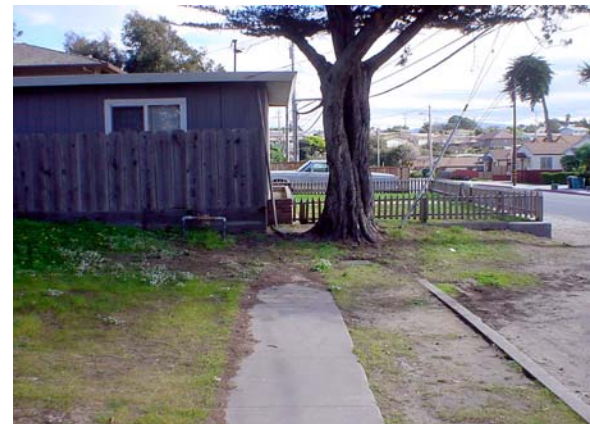
Typical sidewalk gap in Marina
