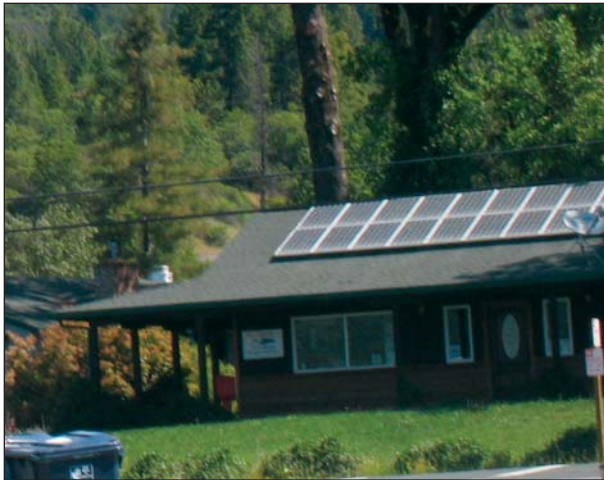
Existing Use of Solar Panels in Laytonville's Town Center
