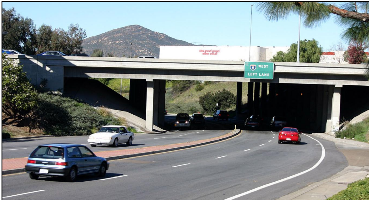
The Jackson Drive undercrossing with narrow and exposed bike lanes and only one sidewalk.
