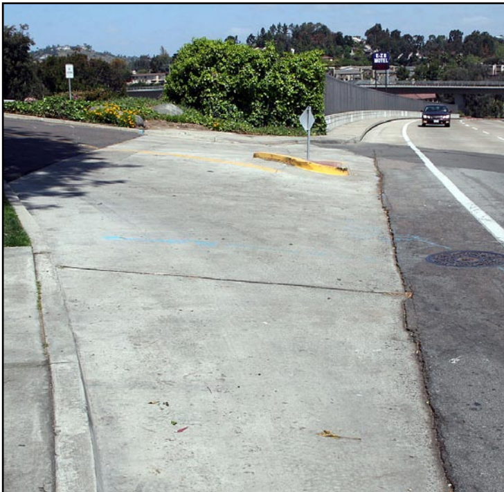
Problem driveway for shopping center near Baltimore crossing.
