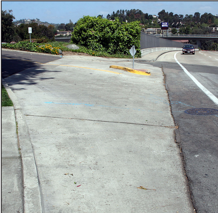
Problem driveway for shopping center near Baltimore crossing.
