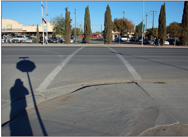
This single ramp at Myrtle Avenue does not align pedestrians with the existing crosswalk.
