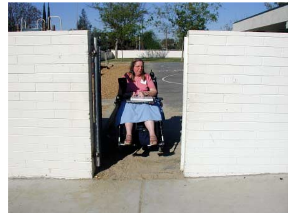
A wheelchair cannot negotiate this entrance to the school grounds because there is a depressed dirt area separating the asphalt on one side of the wall and the concrete on the other side. Neither children nor someone in a wheelchair can see over this wall to determine if it is safe to enter. The area near the school lacks curb ramps and continuous sidewalks.
