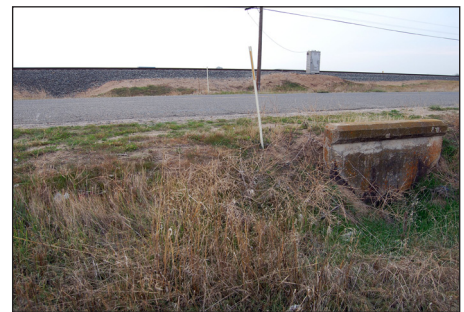
Above, clockwise from top left: Draft Master Drainage Plan; Fairmead's current water system includes two wells, a small treatment system and a storage tank; A filled in culvert that used to provide drainage underneath Fairmead Boulevard and the railroad tracks.
