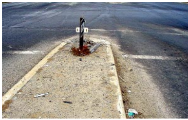
The debris at 416 and 120 indicates this is a site of frequent crashes.
