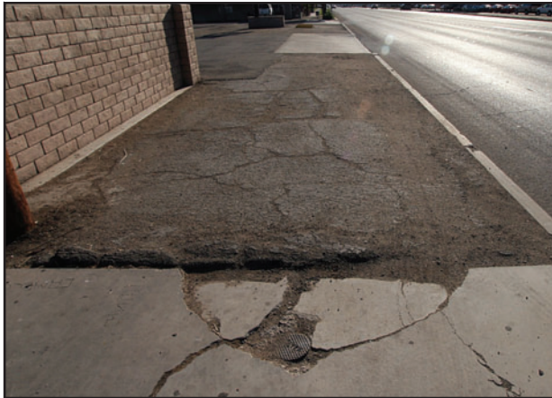
While some sidewalks need repair...
