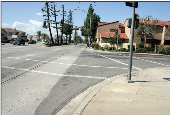
Single pedestrian ramps that force wheelchairs and strollers into the turn.
